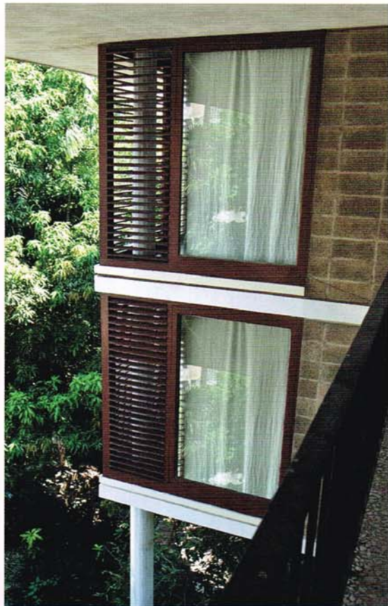
Bottom: As in traditional Havana houses, balconies connect the residents to the life of the street. The louver walls can be slid away to incorporate this outdoor space into the core of the house.
